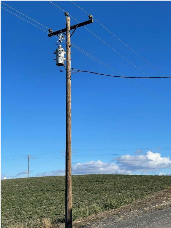
Single-phase transformer with overhead service
