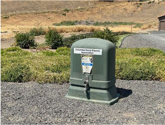
Secondary (120/240 volt) junction box
