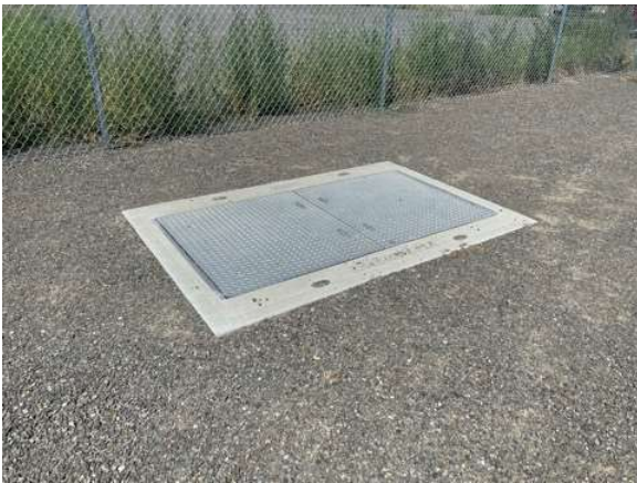
Primary (14,400 volt) vault 5ft W x 7ft L
