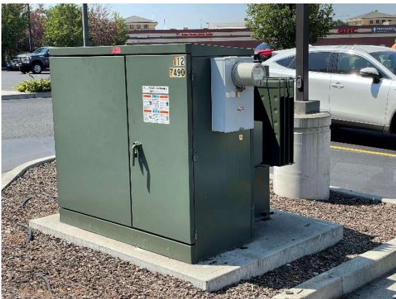
Three-phase transformer with CREA meter
