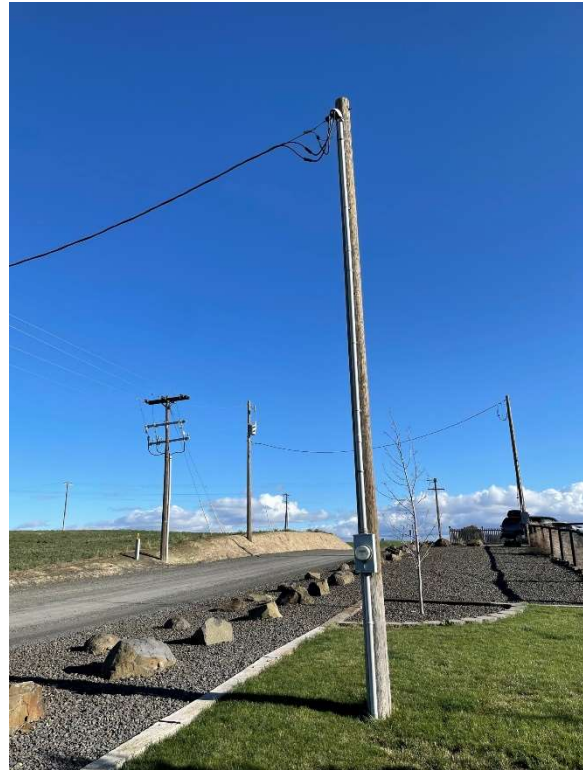
Meter pole and meter base
