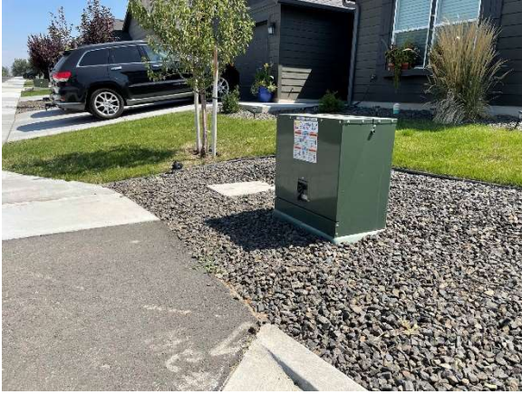
Single-phase primary (14,400 volt) junction box
