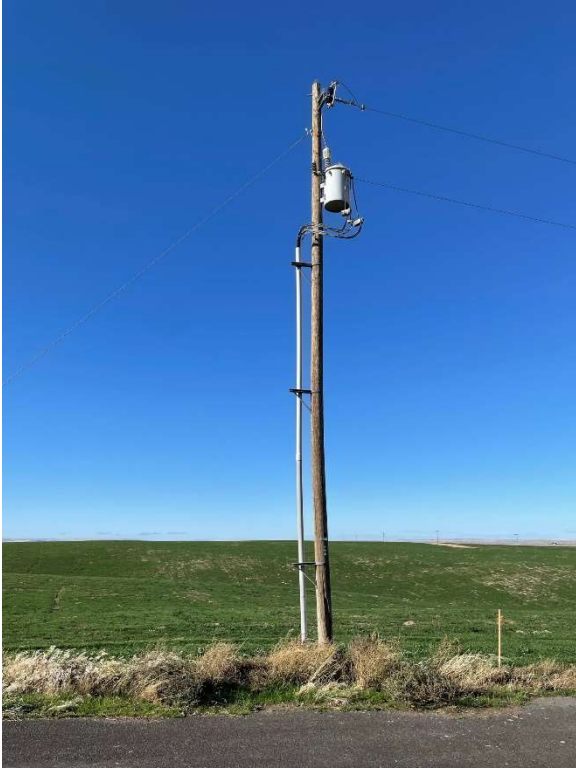
Single-phase transformer with underground service
