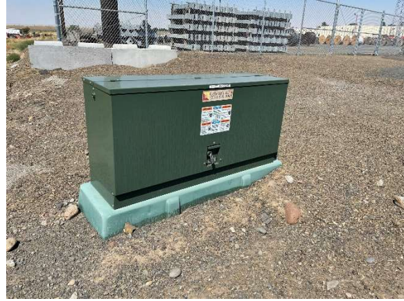
Three-phase primary (14,400 volt) junction box
